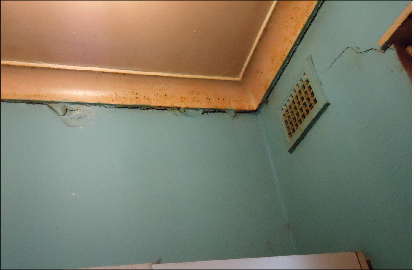
7.1 Kitchen/Dining. Badly needs painting
