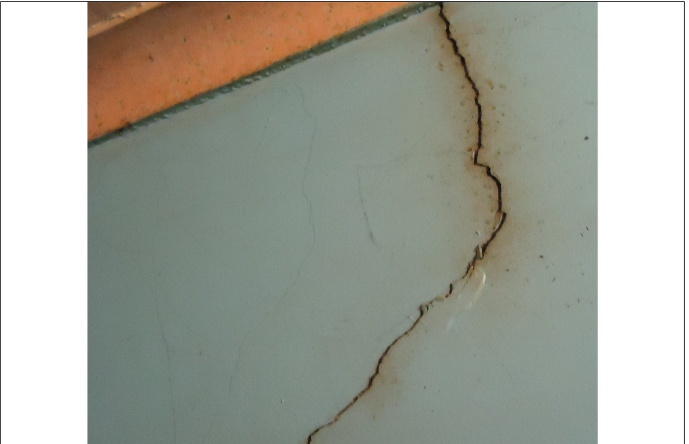
6.2 Kitchen/Dining wall. One of three cracks.
