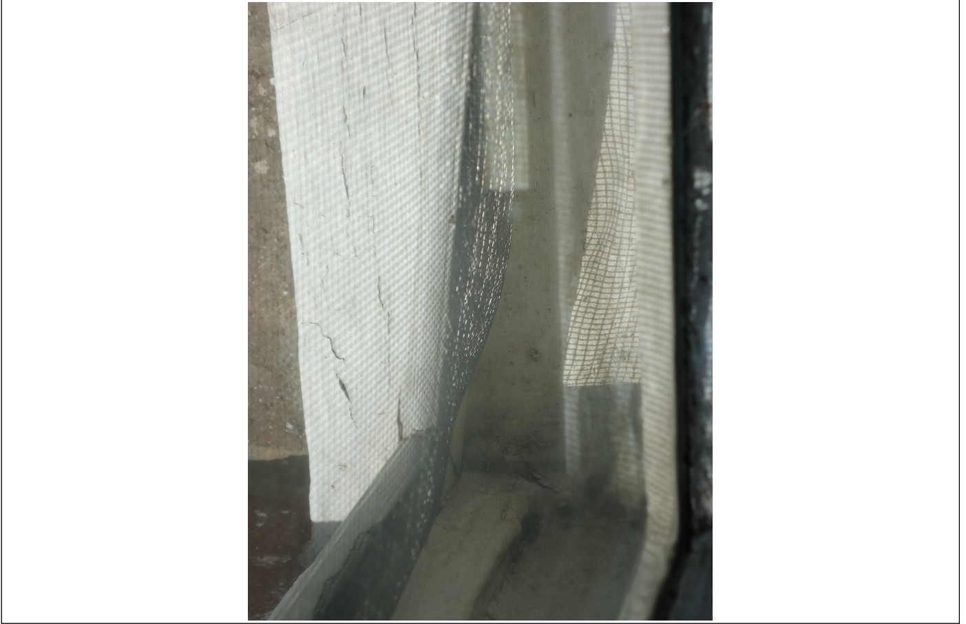
9.1 Living room Window 1. Opens but flyscreen does not fit. Badly needs repair & paint.
