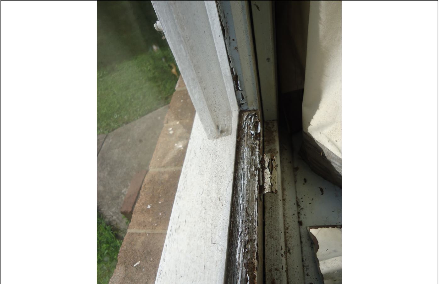
9.2 Living room Window 2. Badly needs repair and paint. No flyscreen.
