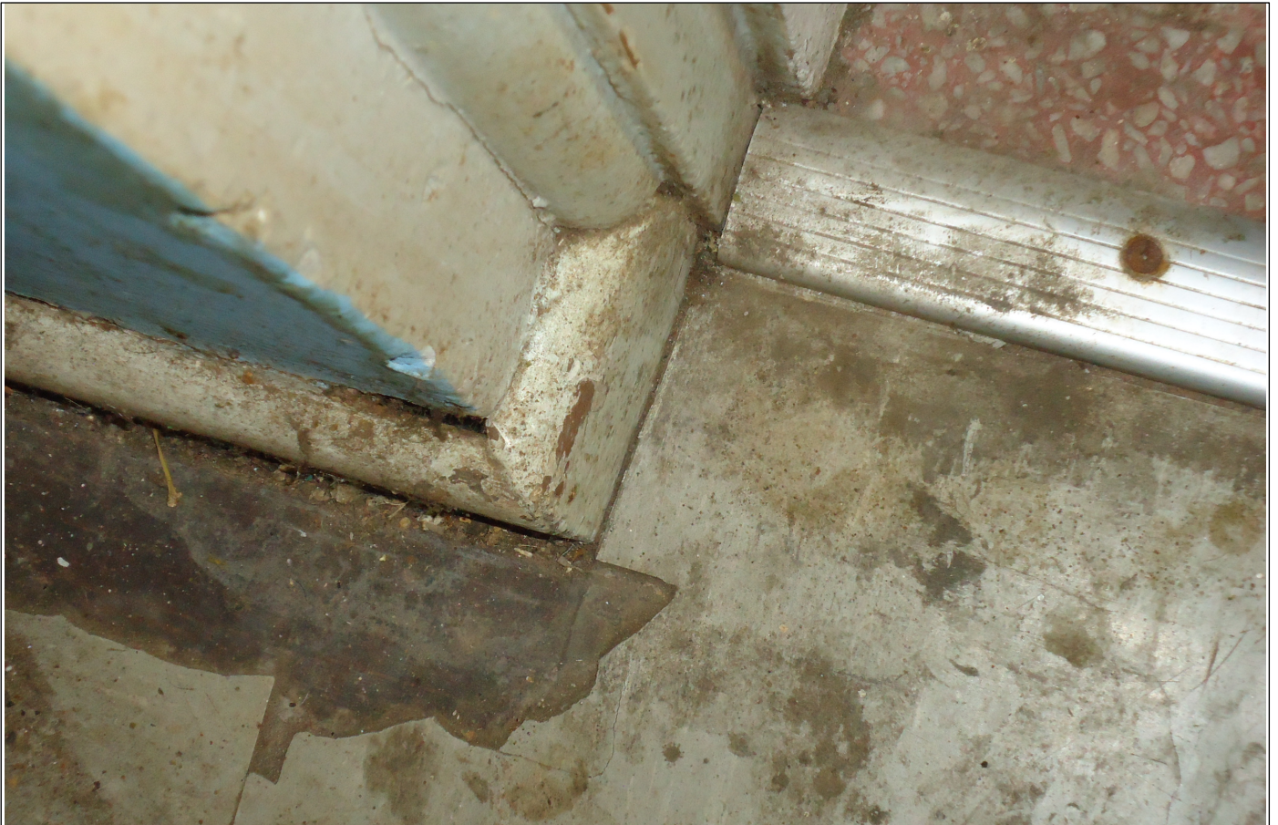
7.2 Kitchen Linoleum back door. Tiles missing. The finish has worn away, the dirt sticks, the linoleum cannot be cleaned.
