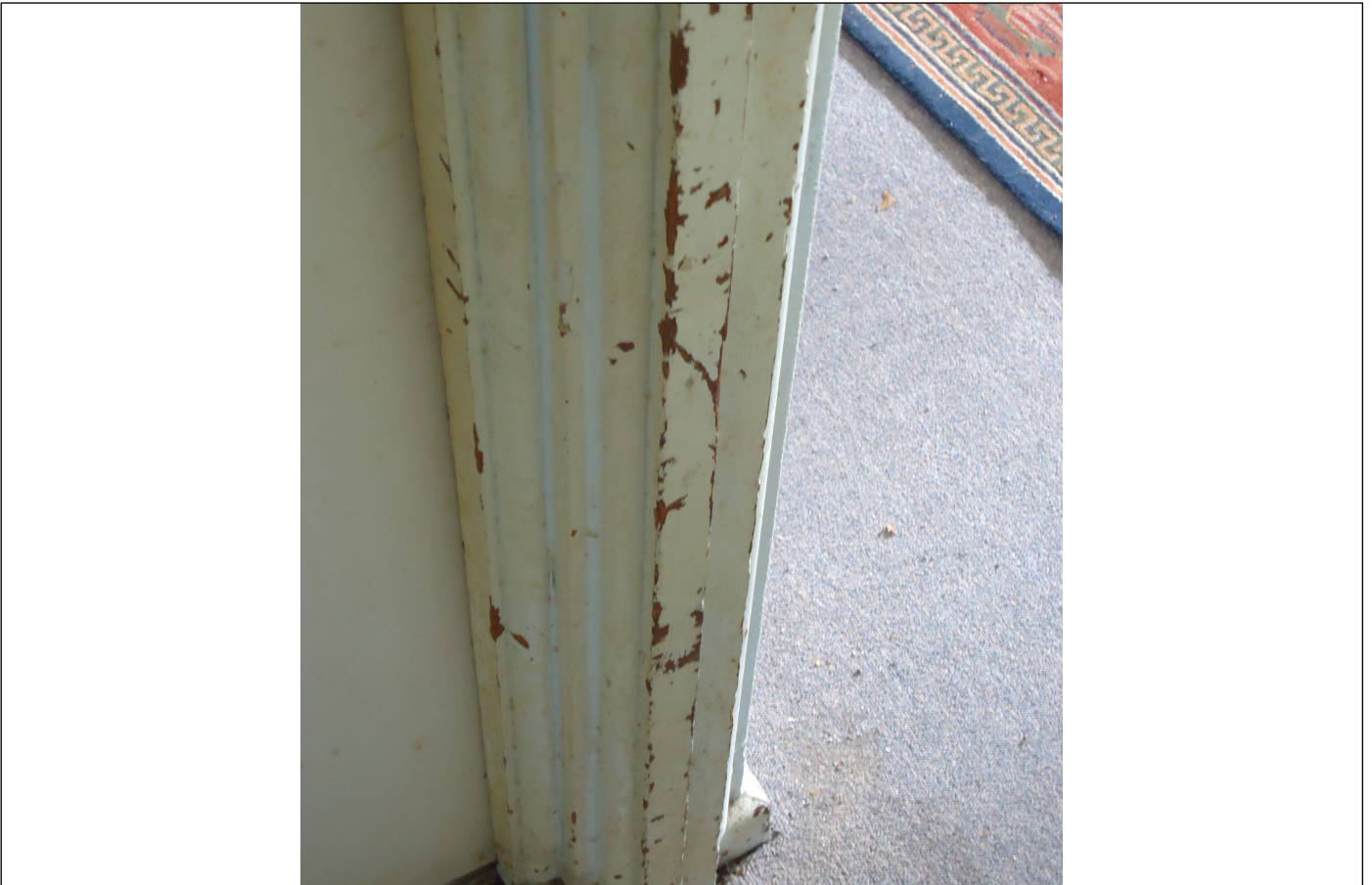
10.2 Living room entrance. Badly needs paint.
