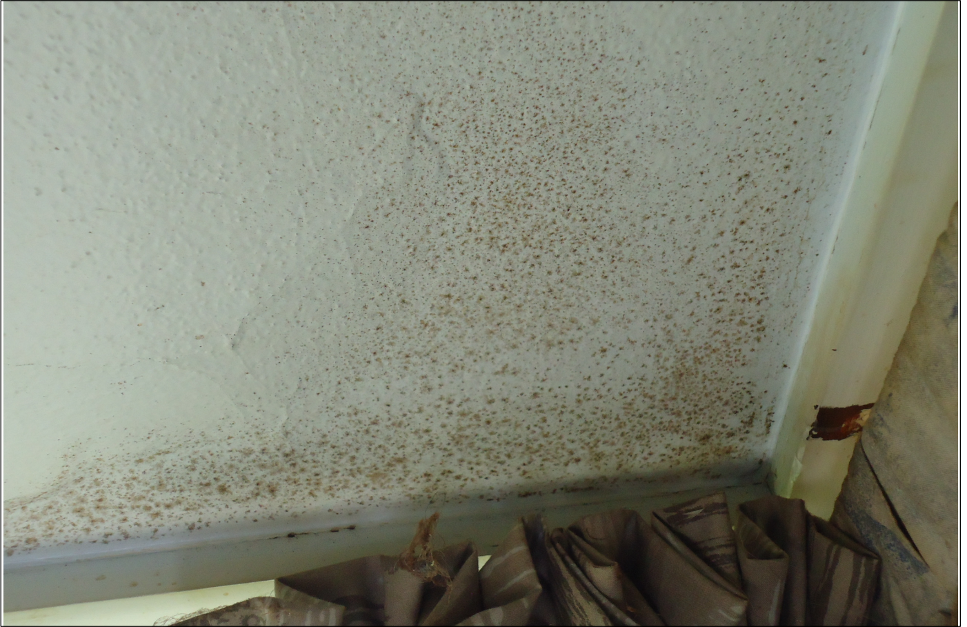
10.1 Living room Ceiling. Damaged, needs paint.
